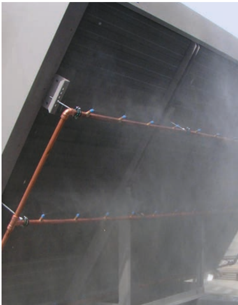
Fig. 2 View of a dry/wet cooler with water spray outwards
