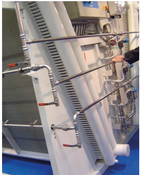
Fig. 3 View of dry/wet cooler with water spray inwards
